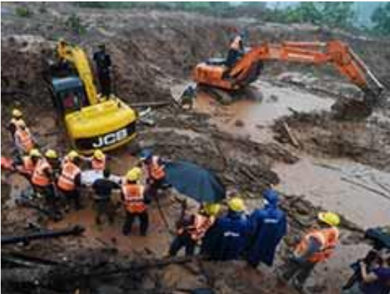
Figure 1 Rescue team working hard to remove the people buried under the clay.
